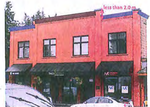
The purple and blue lines above represent the roofline. The blue lines indicate the main roofline while the purple line indicates the parapet or false roof.
