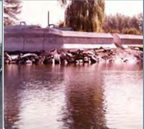
Concrete Cribbing which replaced earlier wooden cribbing in the 1970s | City of Courtenay
