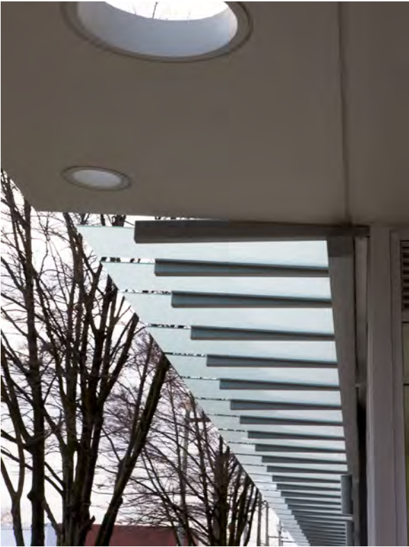
Example of a continuous weather protection option, such as along exterior building walls directly adjacent to pedestrian networks and areas (guideline 59).
